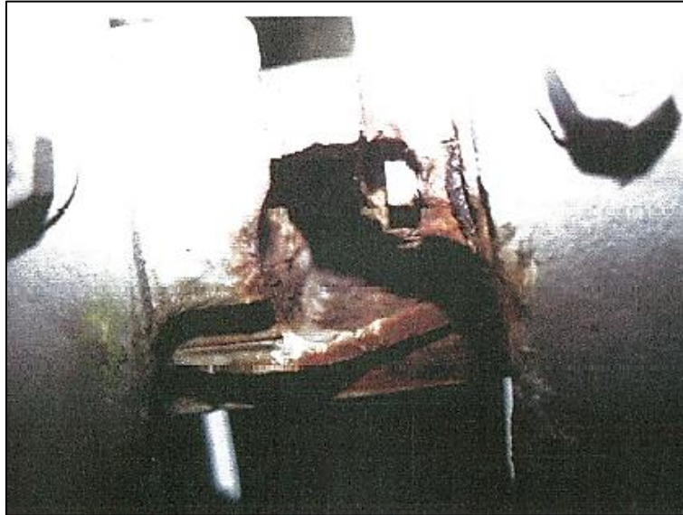
Figure A- 5: Corrosion to bearing plates at central pin from beneath pin area (1996).
