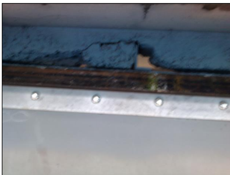
Figure A- 8: Concrete breakdown around shear connectors (2014)
