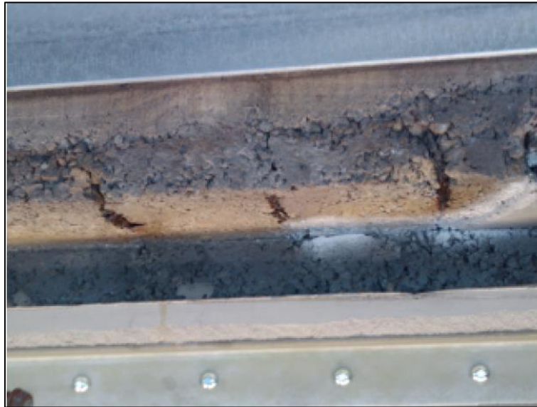
Figure A- 7: Exposed reinforcement and honeycombing in deck (2014).
