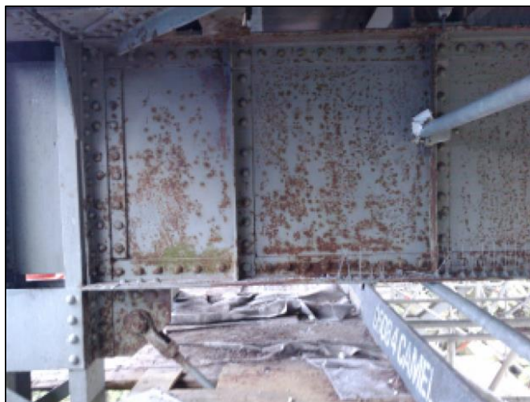
Figure A- 9: Typical corrosion blistering on transverse beam (2014).
