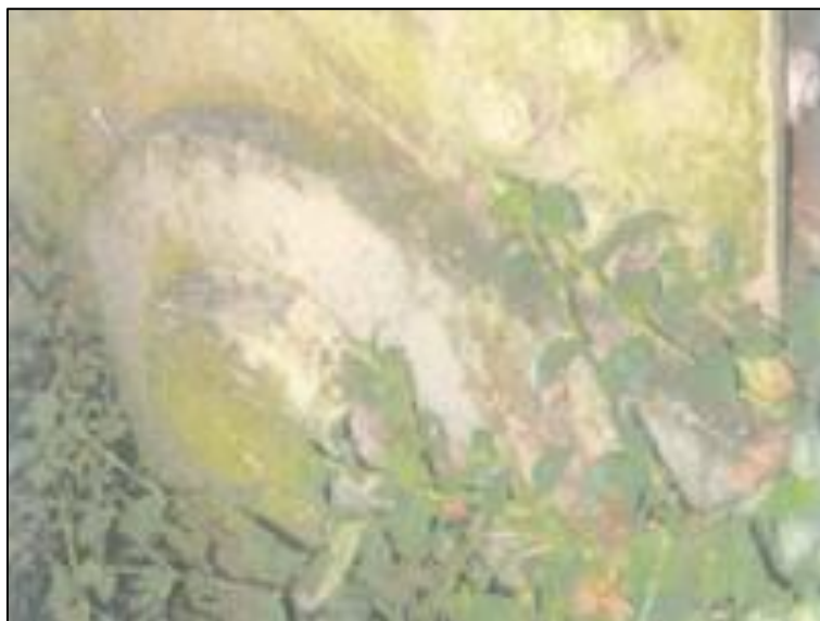
Figure A- 6: Algal growth around pin support at Pier C (2012).
