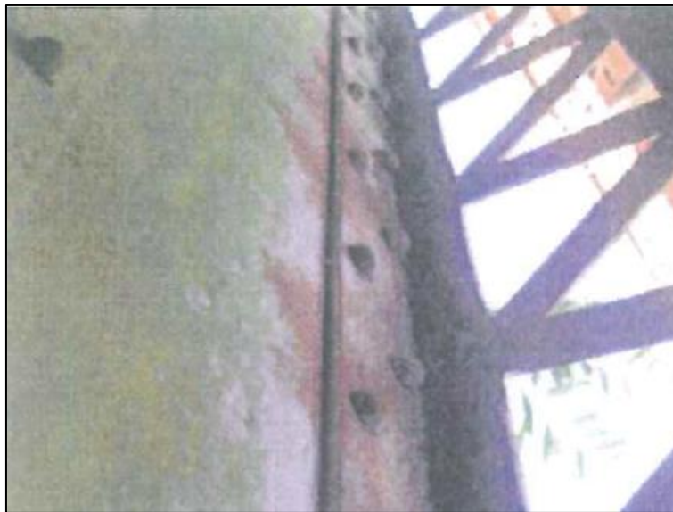
Figure A- 1: Surface corrosion inside lattice column at Pier C (2012).
