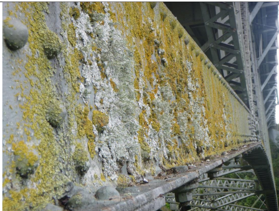
FUNGAL GROWTH ON INTERNAL FACES OF LACED COLUMN
