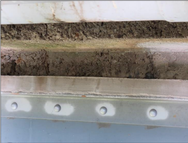
Figure 4-18 - Honeycombing and exposed reinforcement in deck
