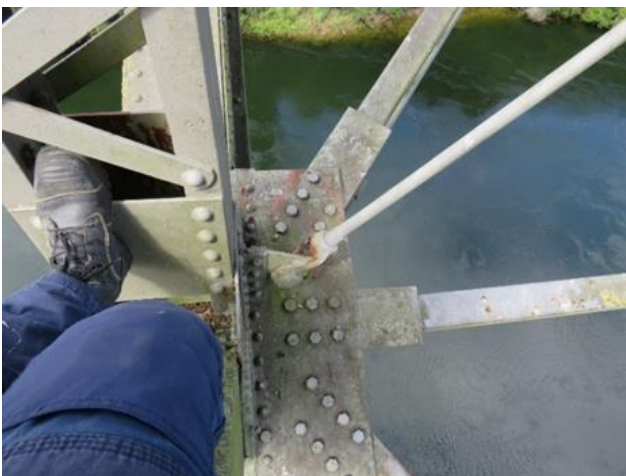
Figure 4-1 Corrosion at bracing connection at UT4.
