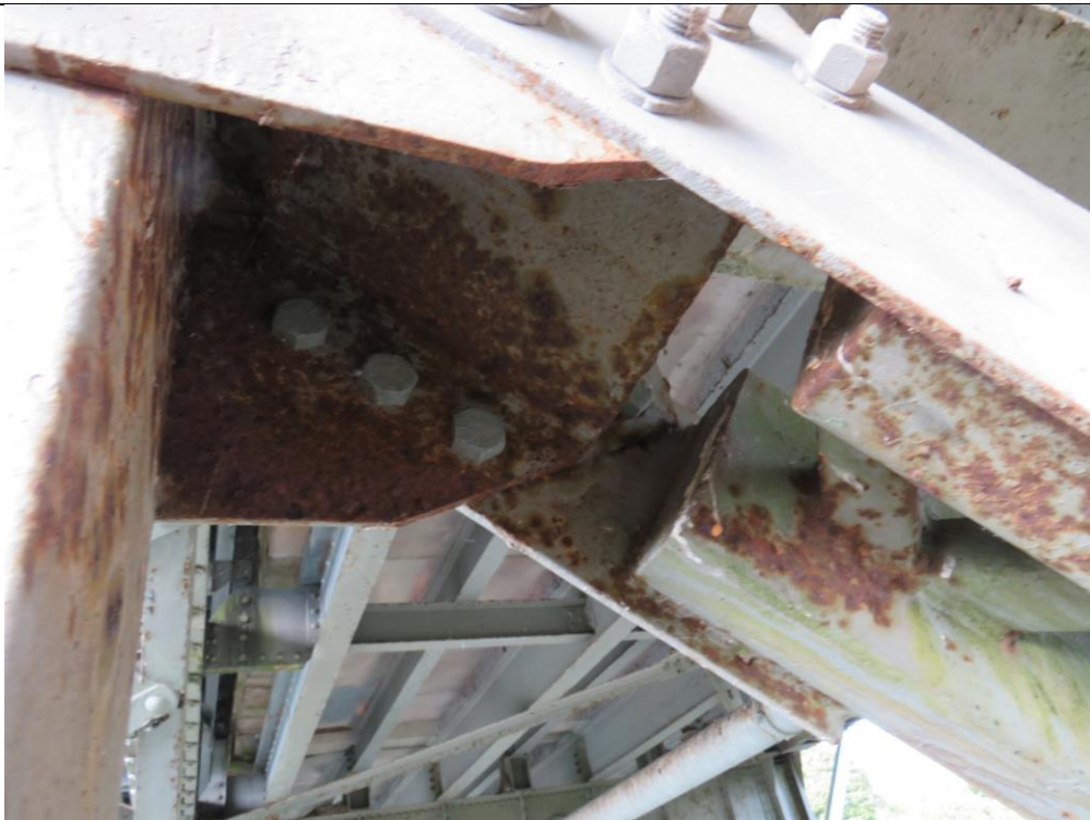
SURFACE CORROSION AT CONNECTION NODE OF DIAGONAL CROSS BRACING
