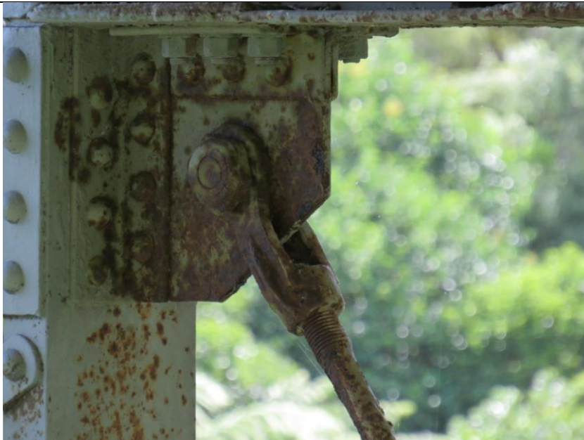
GENERAL COROSION WITH METAL LOSS AT TENSION STIFFENER CONEECTION
