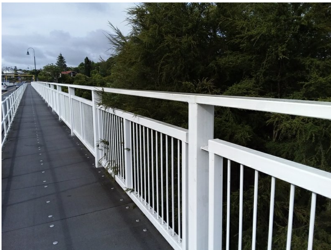
Guardrail / Handrail / Safety Fences (Element 22): Overgrown vegetation at footpath handrail. Downstream at L/10 from Cambridge end.
