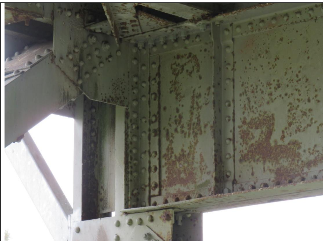
SURFACE CORROSION SCATTERED ON TRANSOM
