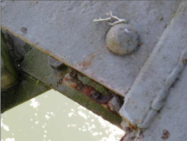
Figure 4-7 - Full penetration corrosion at UB11
