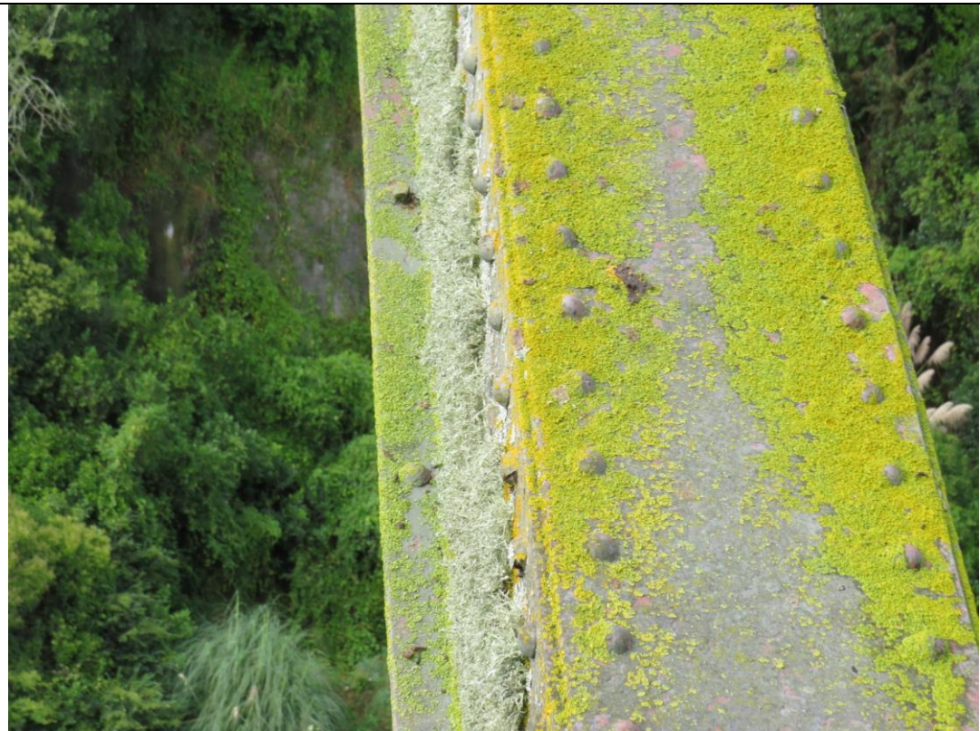
FUNGAL GROWTH WITH CORROSION VISIBLE AT RIVET ENDS
