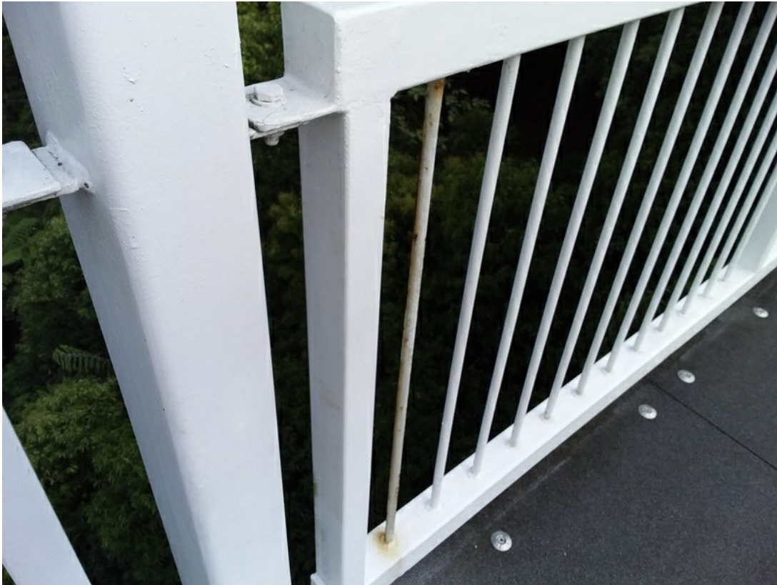
Painting: Barriers / Guardrails (Element 20): Loss of coating on traffic barrier. Downstream at L/6 from Cambridge end.
