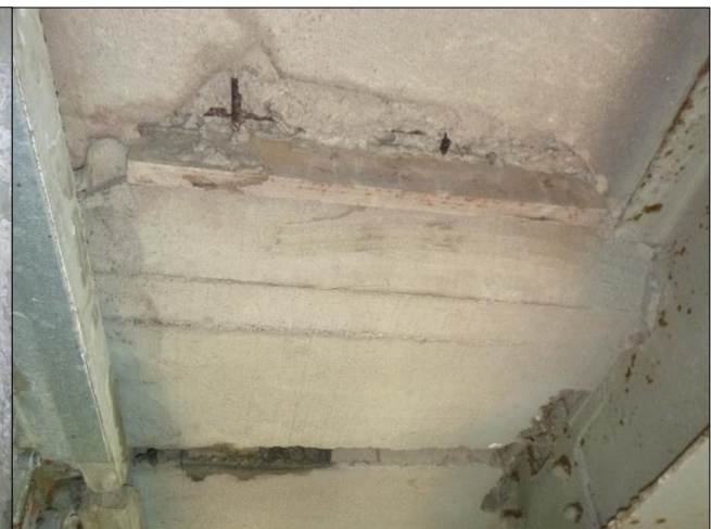
Figure 4-21 - Spalls adjacent to expansion joints at UP Span 6-7 T2-3.
