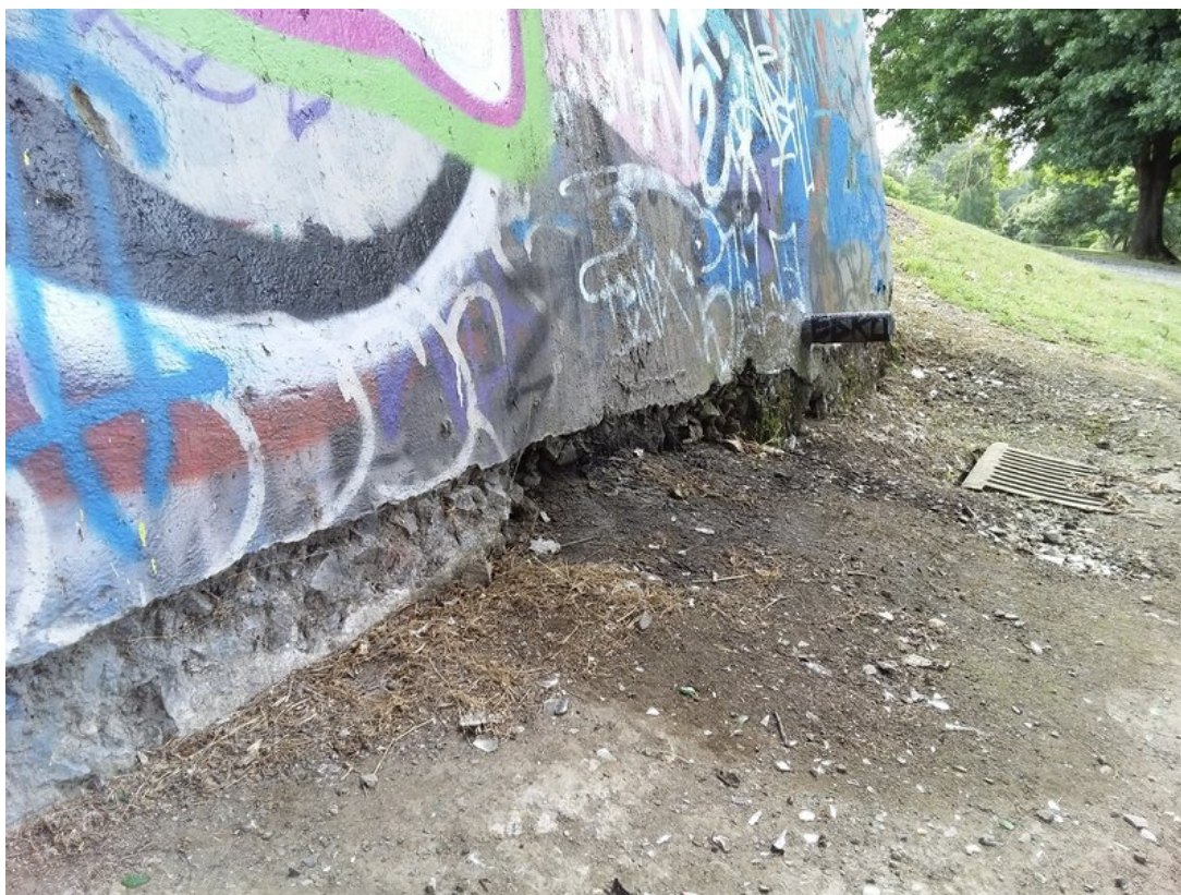
Scour (Element 29): Erosion at base of upstream side of Abutment A caused by stormwater runoff.
