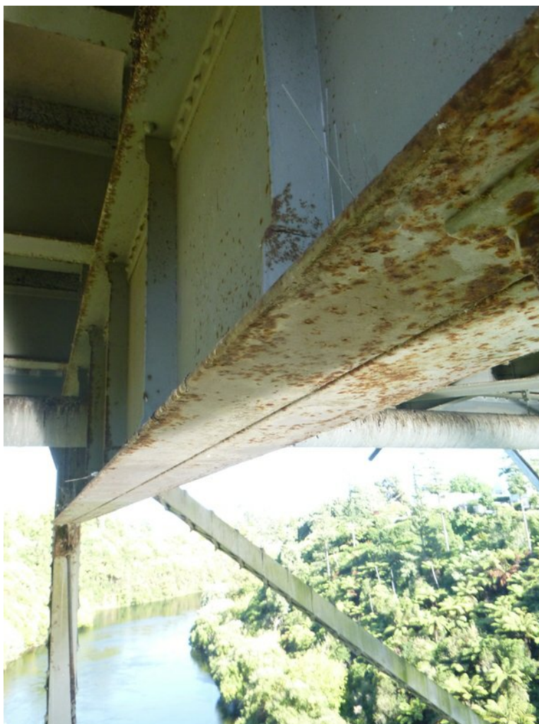
Secondary Elements - Transverse Beams (Element 2): Widespread corrosion spots were observed on element "UT09-DT09".
