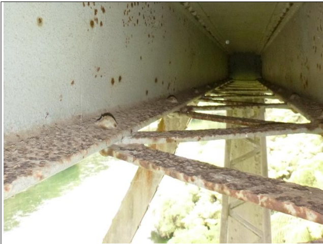
Figure 4-5 - Corrosion to lacing of Transom UT01-DT01
