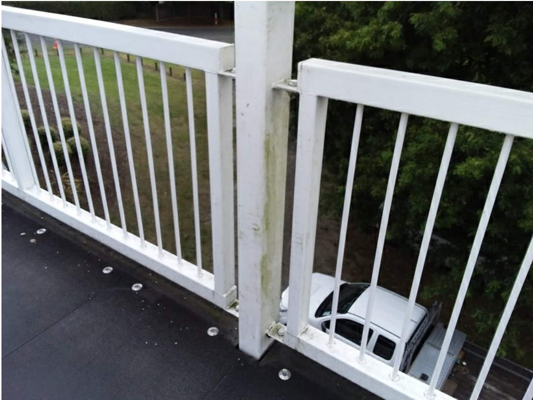
Painting: Barriers / Guardrails (Element 20): Moss growth on footpath handrail posts. Worst over the land spans.
