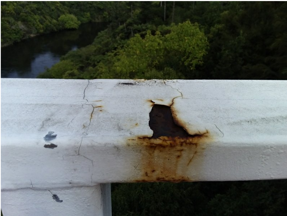
Painting: Barriers / Guardrails (Element 20): Loss of coating on top of footpath horizontal capping rail. Downstream at L/10 from Cambridge end.
