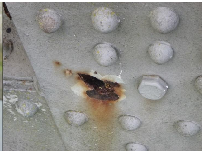
Figure 4-10 - Deep corrosion at UB08
