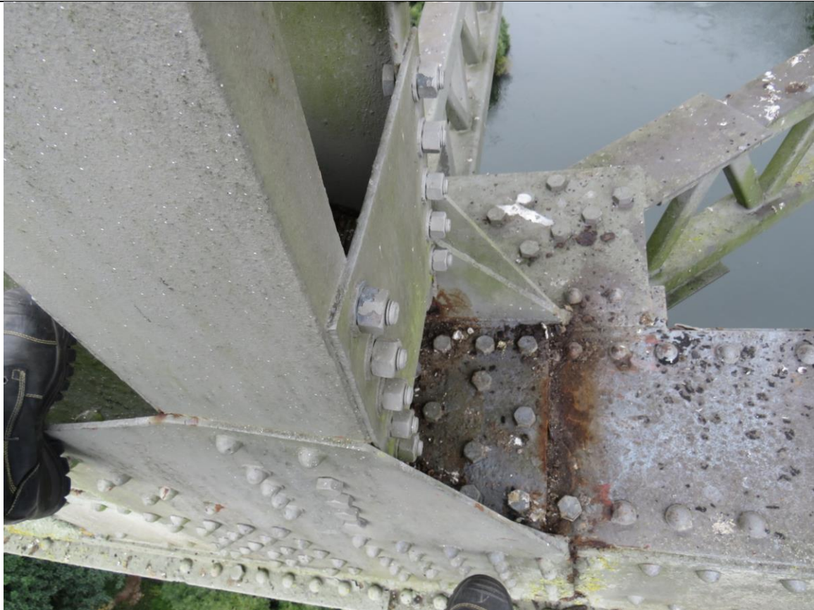
GENERAL CORROSION AT VERTICAL COLUMN AND ARCH CONNECTION
