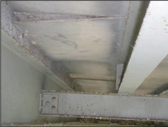
Figure 4-22 Loose, broken and missing asbestos panels observed on all bays at UP Span 5-6 T2-3.
