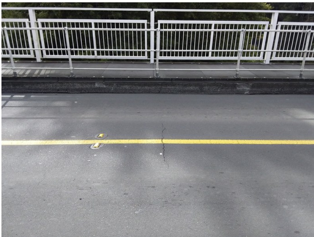
Carriageway Surfacing (Element 23): Transverse cracking on surfacing at 12m from Abutment A.
