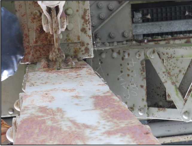
Figure 6-1 General corrosion and loss of paint
