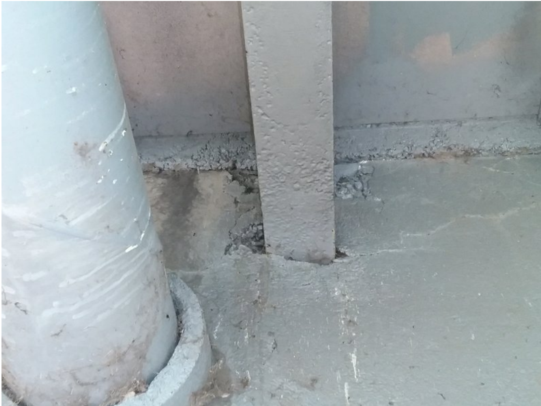
Abutments (Element 9): Loose concrete on face of Abutment B at ends of Stringer 4.
