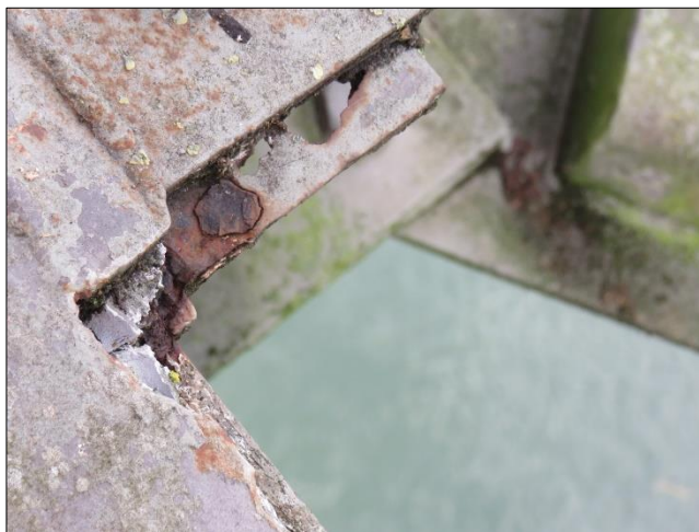
Figure 4-9 Full penetration corrosion at UB03
