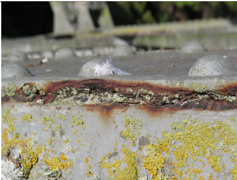
PITTING CORROSION WHERE JOINT SEAL HAS FAILED.
