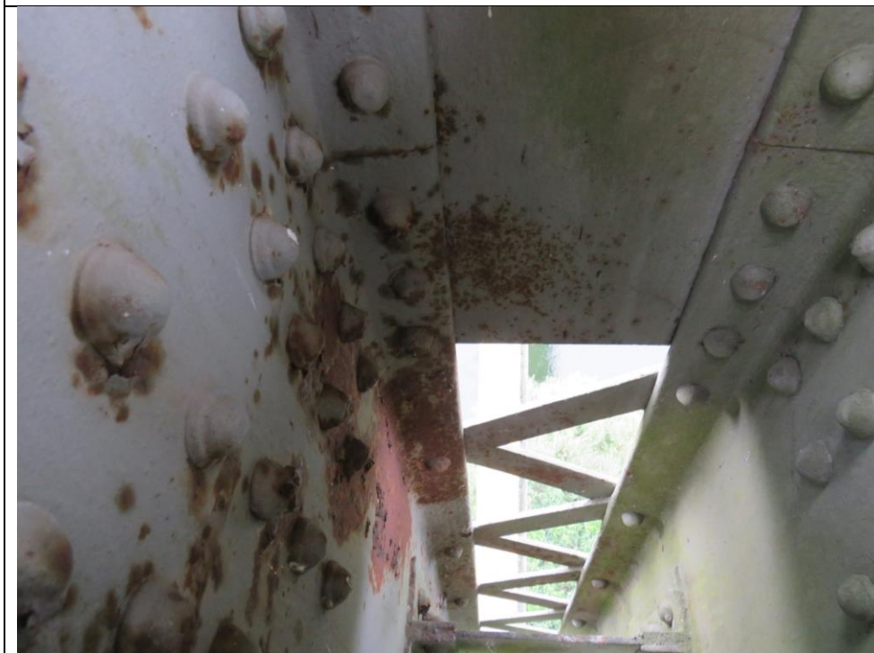
CORROSION ON INTERNAL FACE OF VERTICAL LACED COLUMN CAUSING COATING DELAMINATION
