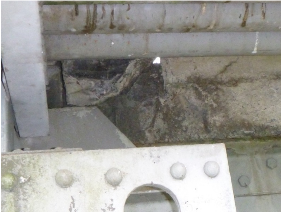
Superstructure Drainage (Element 15): Void in kerb allowing water to drain onto steelwork at Span DE.
