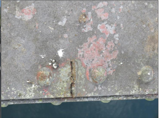
Figure 4-12 - Steel crack in arch chord UB05-UB06, likely historic, monitor.
