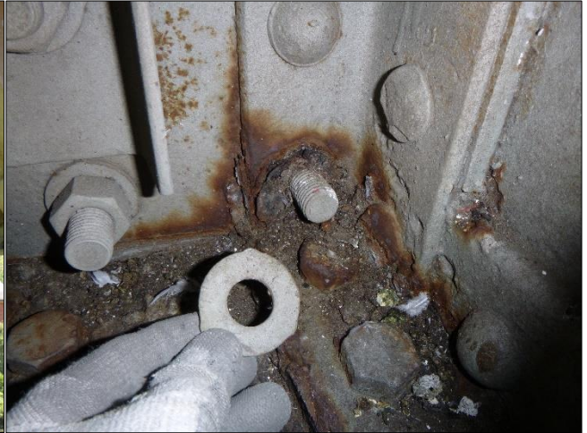
Figure 4-4 - Nut missing on transom at T10.
