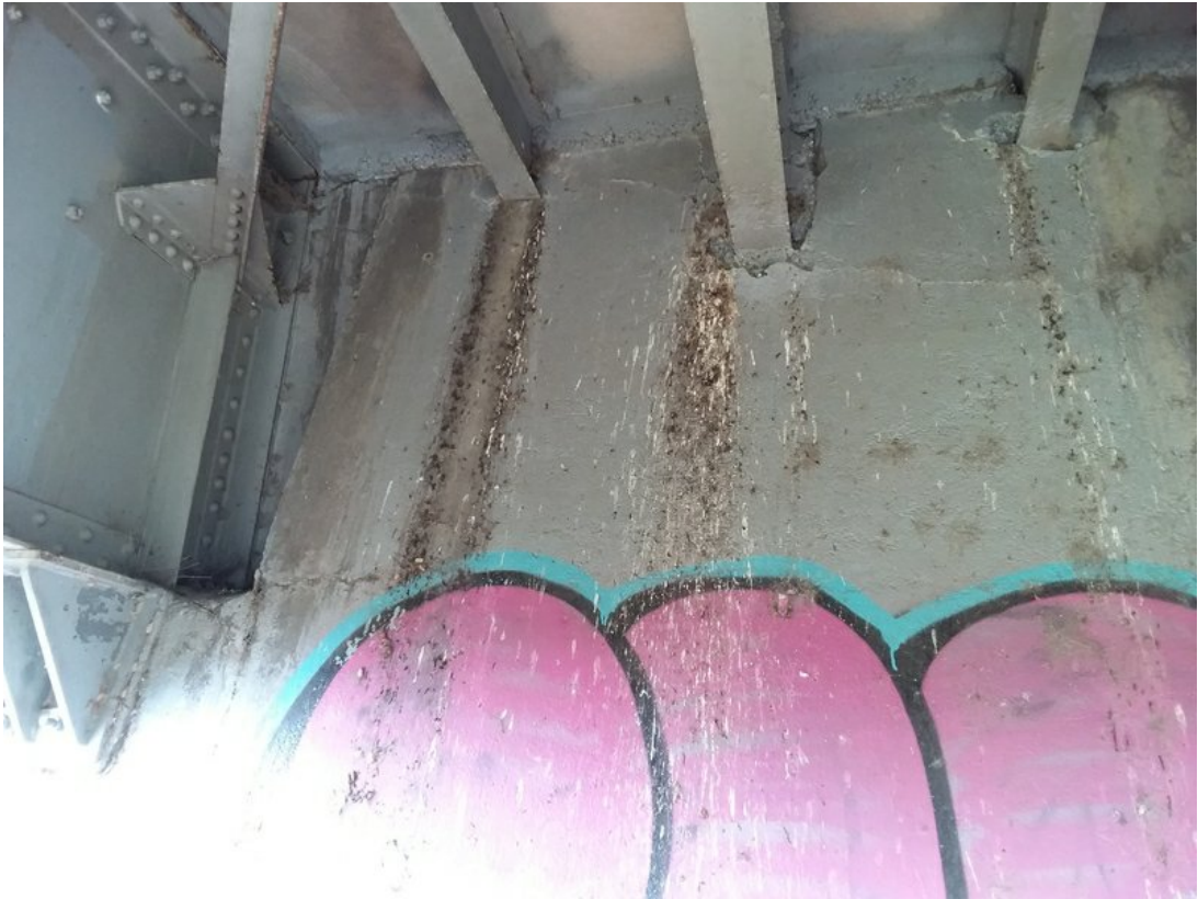
Substructure Drainage (Element 16): Water leakage marks on front face of Abutment A.
