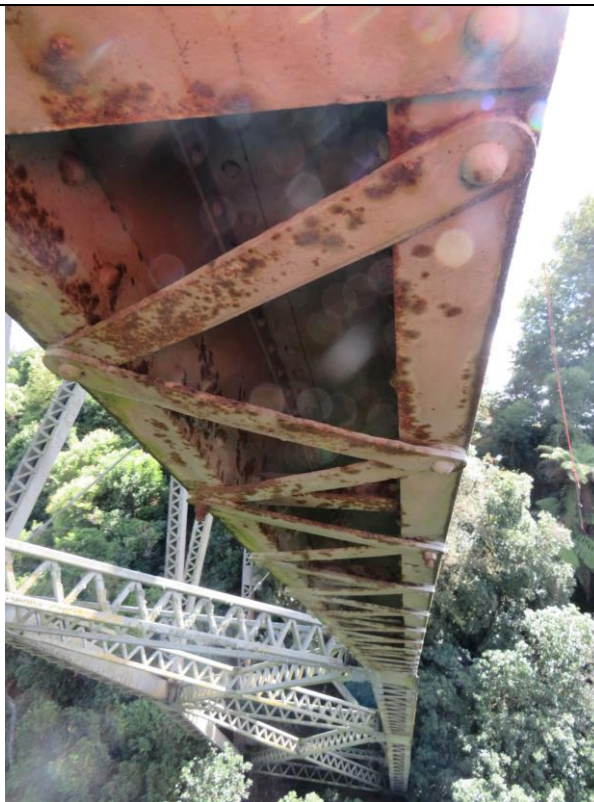
GENERAL CORROSION ON UDESIDE FACE OF BOTTOM ARCH
