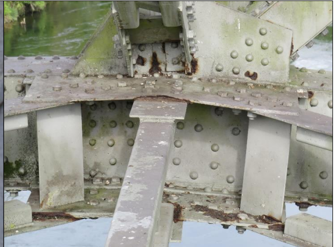
Figure 4-8 - Plate is bent with corrosion present on underside at UT6/DT6.
