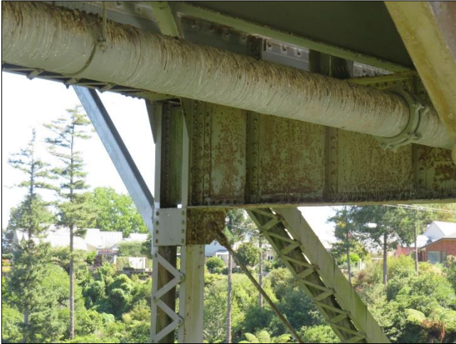
Figure 4-3 - Widespread corrosion spots were observed on transom UT09-DT09.
