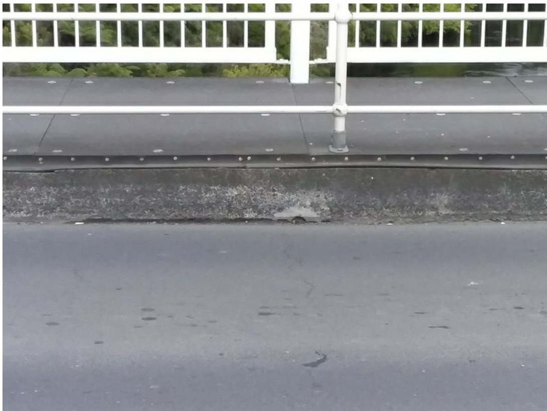
Superstructure Drainage (Element 15): Blocked drain hole on kerb.
