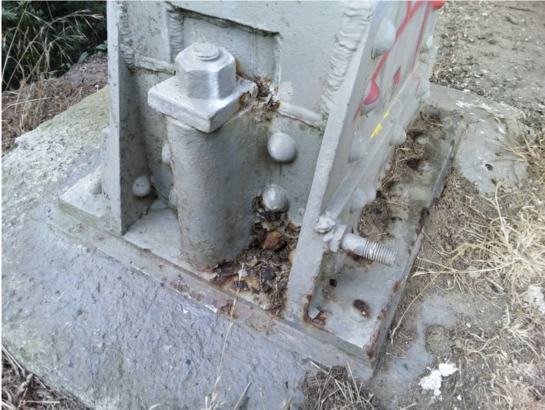
Pier / Column (Element 11): Corrosion on base plate of upstream side of Column Pier B.
