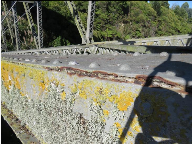
Figure 4-11 - Crevice corrosion in arch chords along top flange to web joint UB09-UB10.
