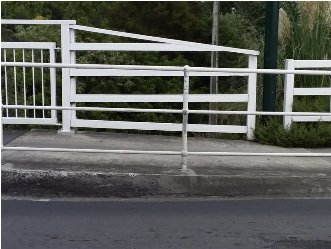
Approach Rails / Barriers / Walls (Element 35): Minor loss of coating on approach barriers. Downstream of Cambridge approach.
