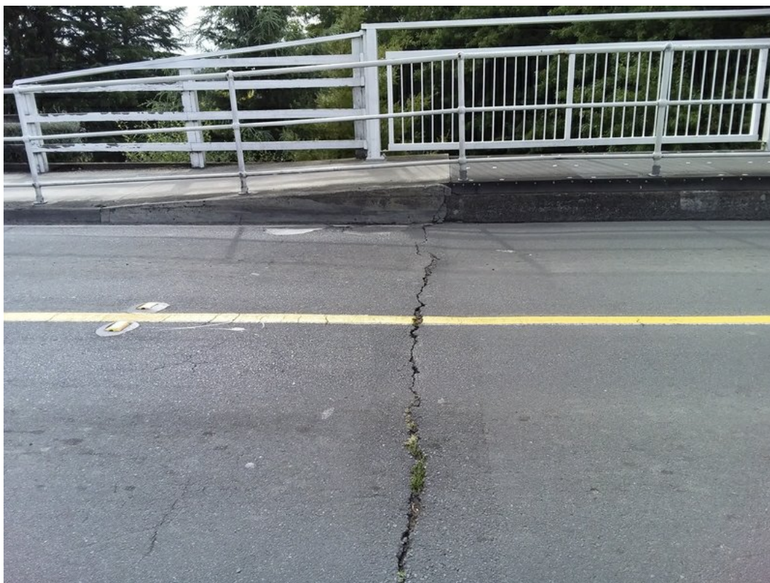
Movement / Expansion Joints (Element 17): Crack to surfacing above Abutment A.
