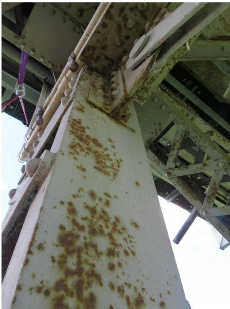
Primary Load Carrying Element (Element 1) : Spots of corrosion on vertical laced columns at UT05.
