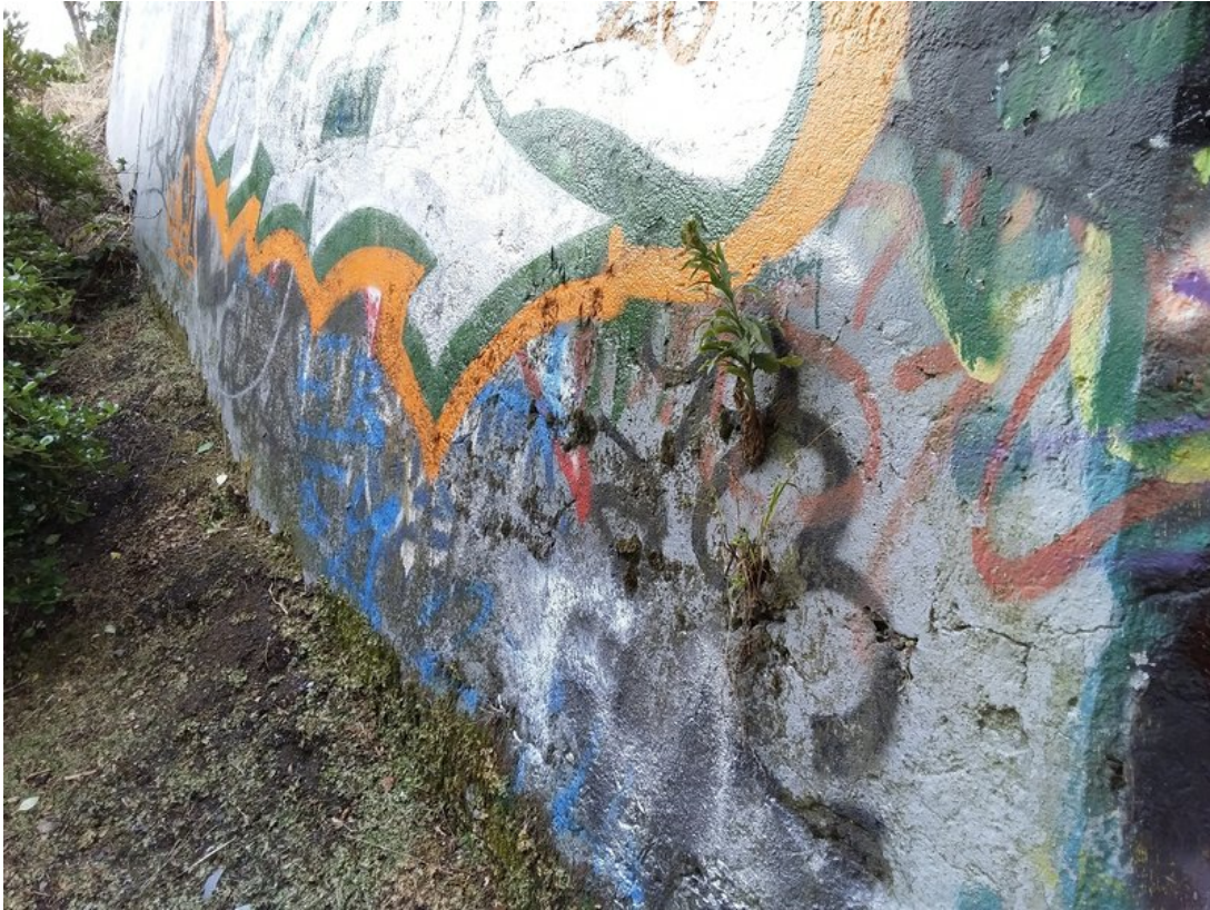
Wing Wall (Element 32): Small shallow void on Approach A downstream wing wall with vegetation growing out of the void.
