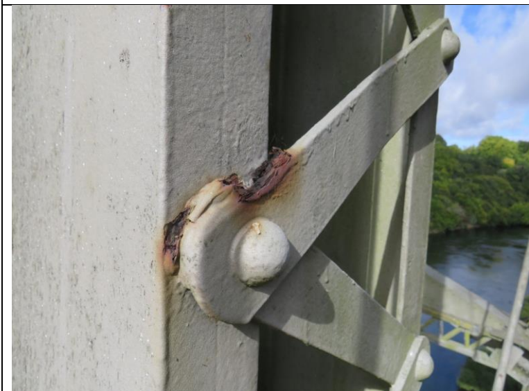
CREVICE CORROSION OF LACE PLATE ON COLUMN
