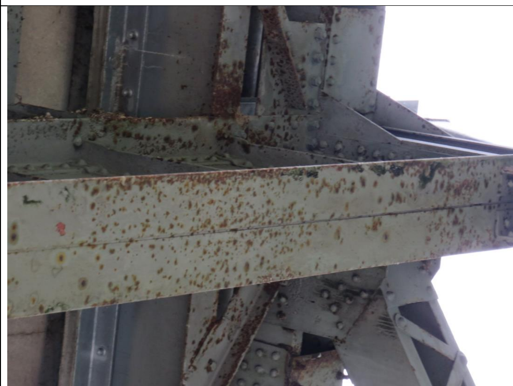
SURFACE CORROSION SCATTERED ON SHARP EDGES AND FLANGE UNDERSIDE OF TRANSOM
