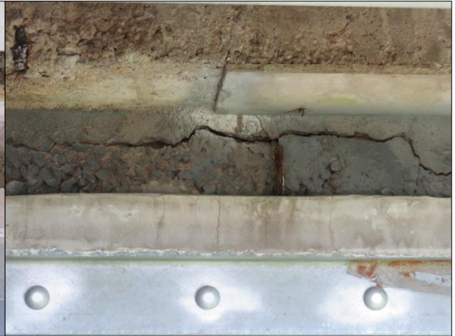
Figure 4-19 - Horizontal cracking in concrete. May be longitudinal shear issue at UP Span 1-2.
