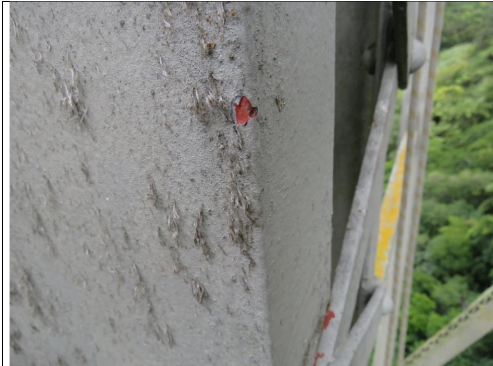
MECHANICAL DAMAGE EXPOSING RED LEAD COATING
