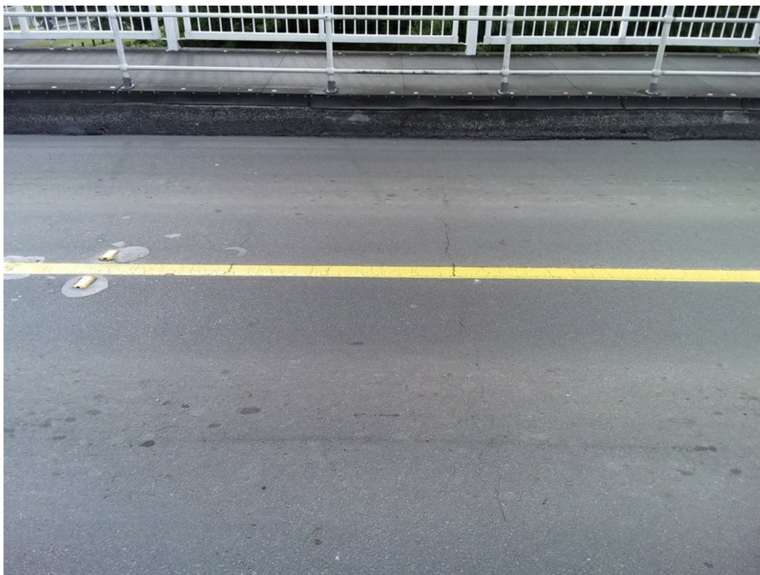
Carriageway Surfacing (Element 23): Transverse cracking on surfacing at 2m from Abutment A.
