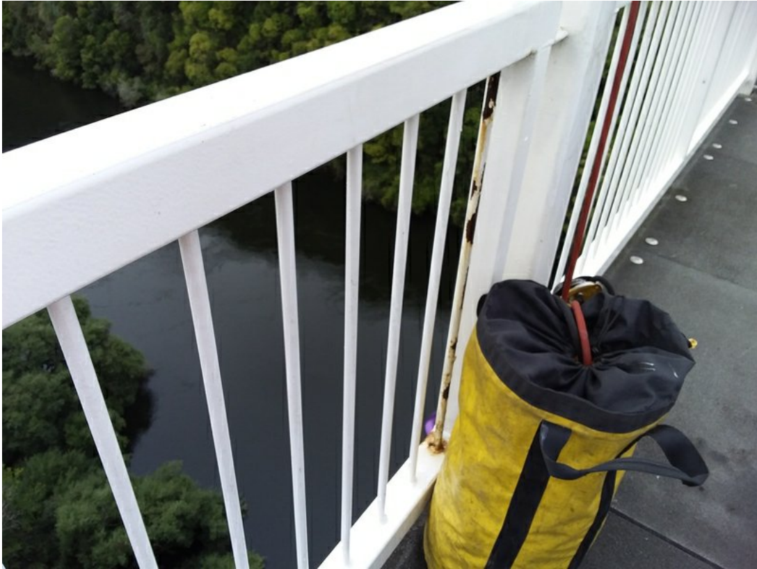
Painting: Barriers / Guardrails (Element 20): Loss of coating on footpath handrail. Upstream at L/5 from Cambridge end.
