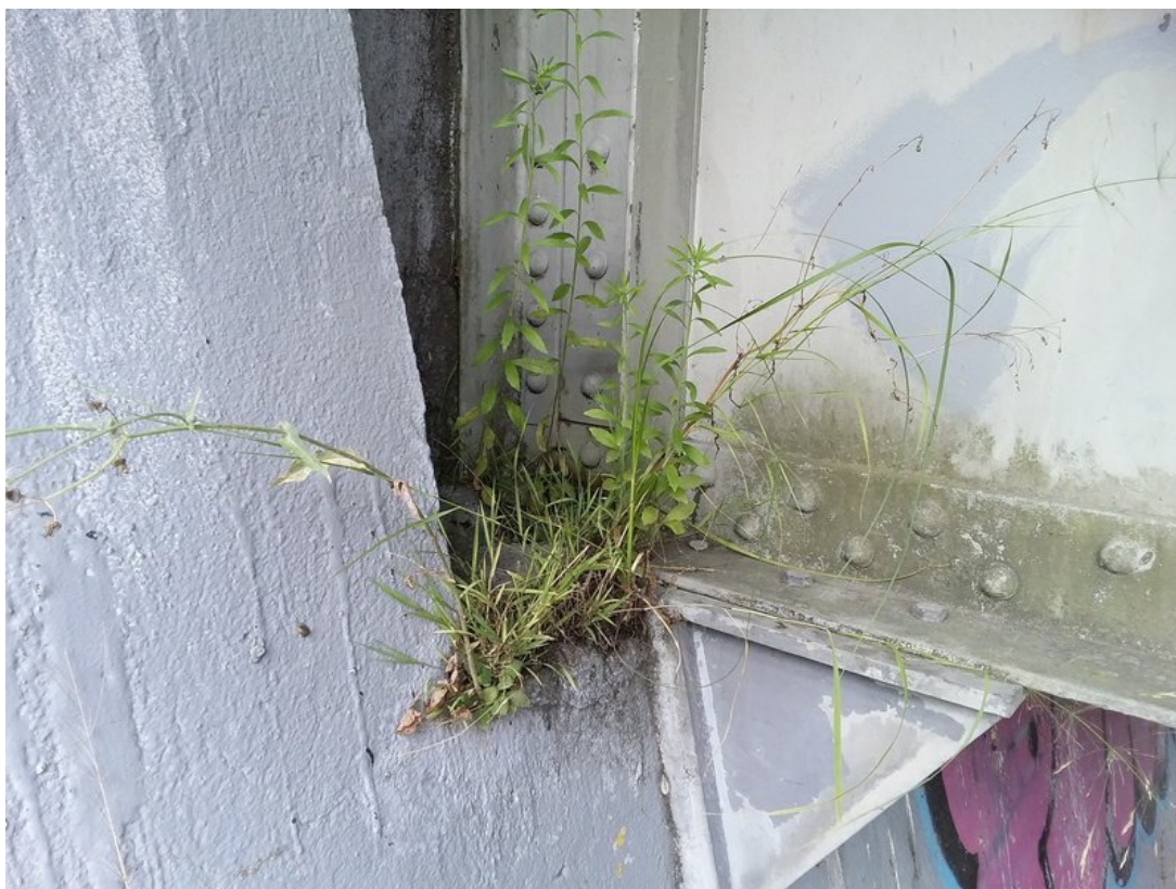
Bearing Plinth / Shelf (Element 14): Vegetation growth on upstream side of Abutment B bearing shelf.
