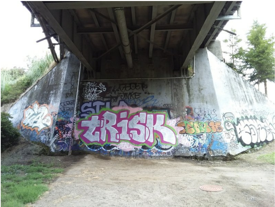
Painting: Substructure Elements (Element 19): Graffiti on Abutment A and wing walls.
