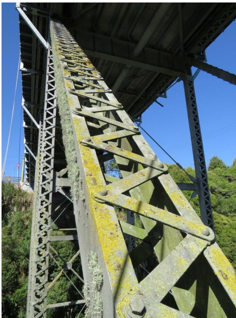
Primary Load Carrying Element (Element 1) : Fungal growth on diagonal laced columns at UT11-UB10.
