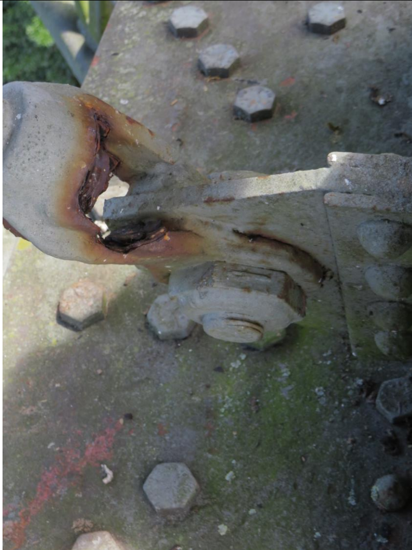
METAL LOSS AT TENSION STIFFENER CONNECTION END
