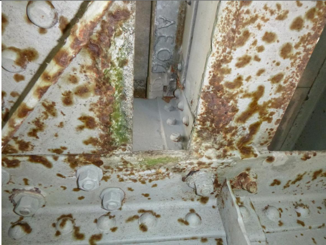
GENERAL CORROSION WITH COATING DELAMINATION AT TRANSOM AND STRINGER CONNECTION
