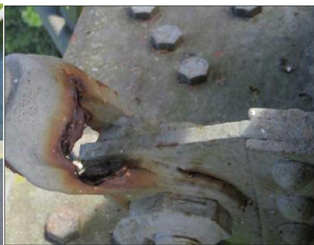
Figure 4-1 - Rod tie at UT4 showing signs of significant corrosion, requires replacement.
