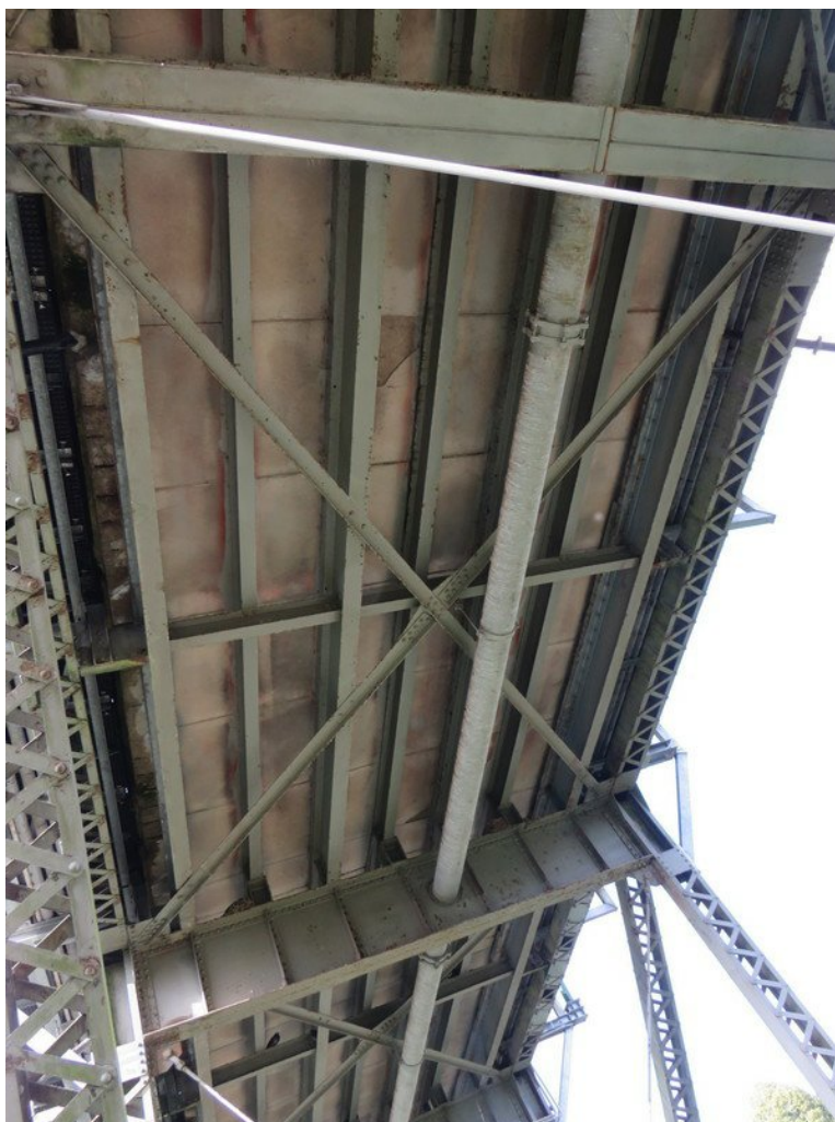
Secondary Elements - Other Including Deck (Element 3): Underside of deck covered by asbestos panels, except where asbestos panels are broken.
