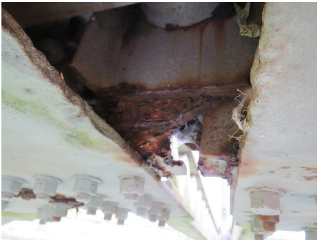
Primary Load Carrying Element (Element 1) : Crevice corrosion, metal loss and coating failure at U/S Centre pin.
