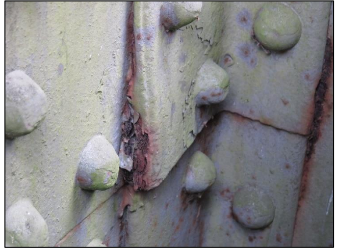
Figure 6-2 Crevice corrosion on edges of elements
