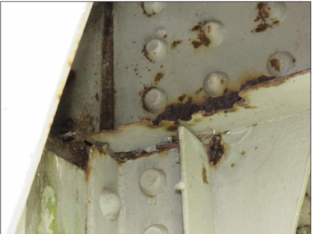
Figure 4-6 - Section loss to bottom flange of Transom UT07-DT07
