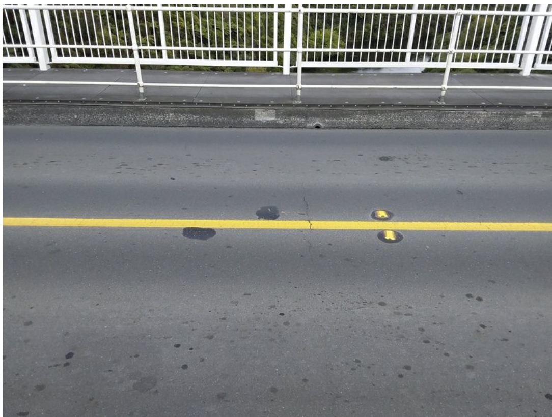
Carriageway Surfacing (Element 23): Transverse cracking on surfacing at 30m from Abutment B.
