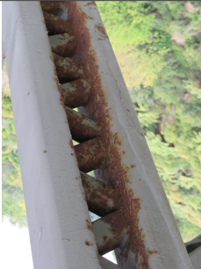
SURFACE CORROSION ON DIAGONAL CROSS BRACING
