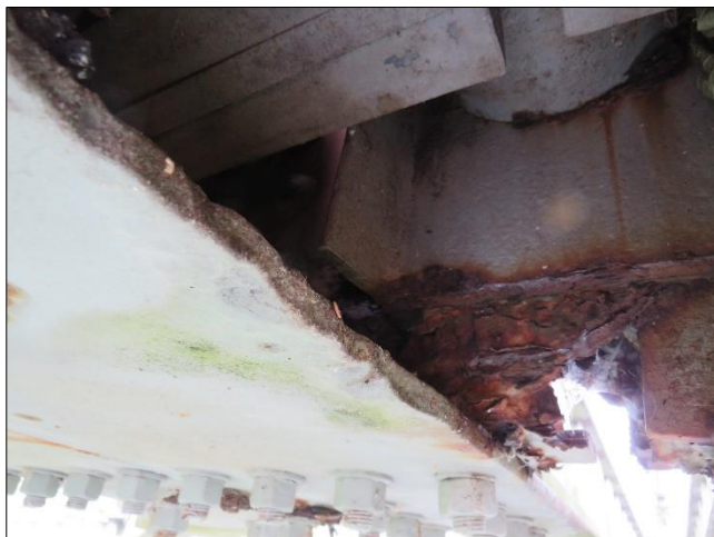
Figure 4-16- Corrosion in steelwork around central pins.
