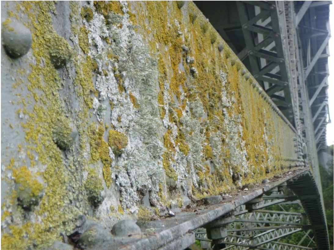
Primary Load Carrying Element (Element 1) : Fungal growth on arch bottom chord at UB07-UB08.
