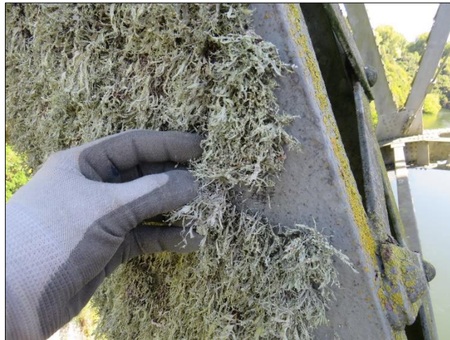
Figure 6-3 - Example of Fungal Growth
