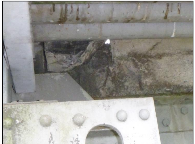
Figure 4-23 – Void in kerb allowing water to drain onto steelwork at Span DE.
