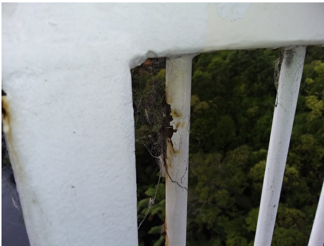
Painting: Barriers / Guardrails (Element 20): Loss of coating on footpath handrail. Upstream at L/5 from Leamington end.
