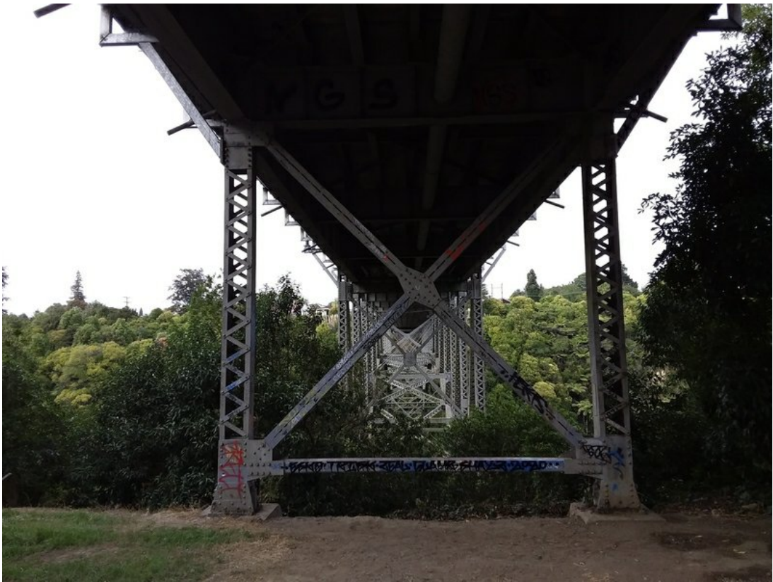
Painting: Substructure Elements (Element 19): Graffiti on A side of Pier B.
