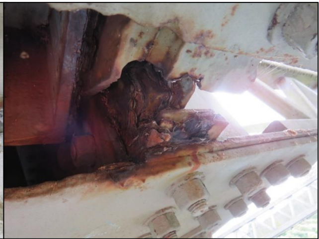
Figure 4-15 - Evidence of significant metal loss at central pins
