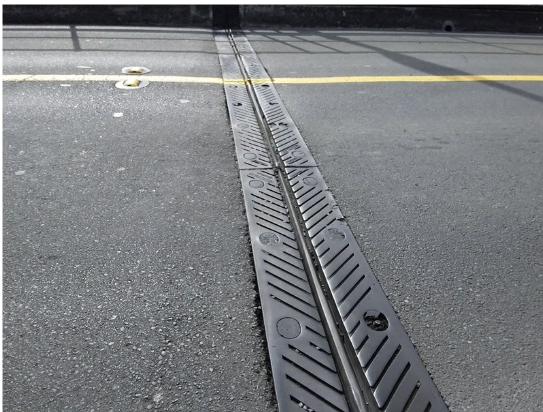
Movement / Expansion Joints (Element 17): Some debris in and around expansion joint.
