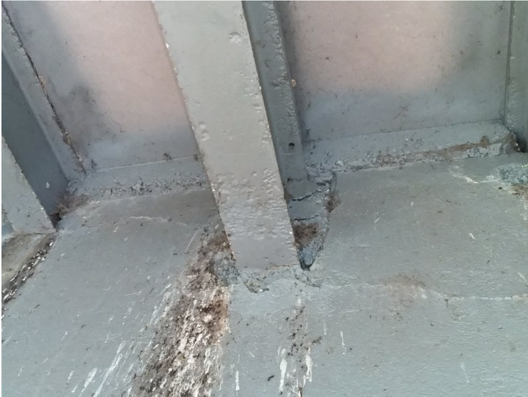
Abutments (Element 9): Loose concrete on face of Abutment B at ends of Stringer 2.
