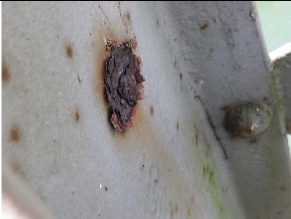
PITTING CORROSION ON INTERNAL FACE OF VERTICAL COLUMN
