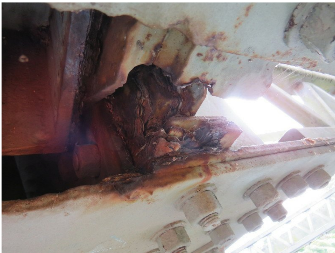
Primary Load Carrying Element (Element 1) : Crevice corrosion, metal loss and coating failure at D/S Centre pin.
