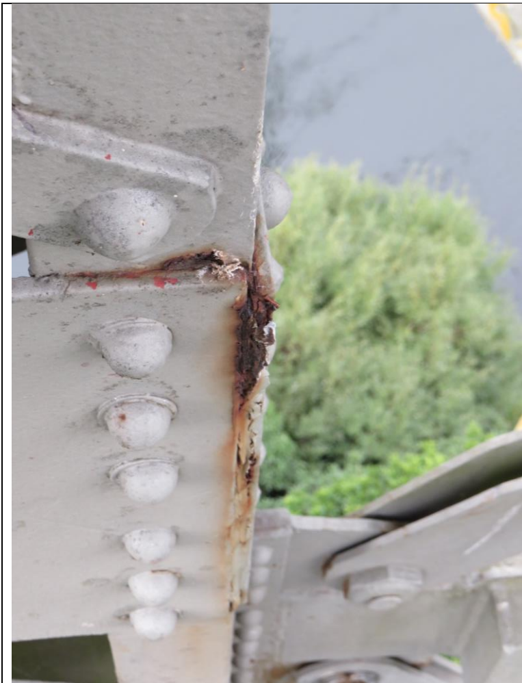
METAL LOSS DUE TO CREVICE CORROSION ON SPLICED SECTION OF LACED COLUMN
