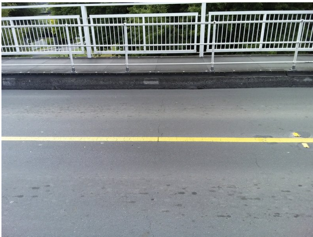
Carriageway Surfacing (Element 23): Transverse cracking on surfacing at 5m from Abutment A.
