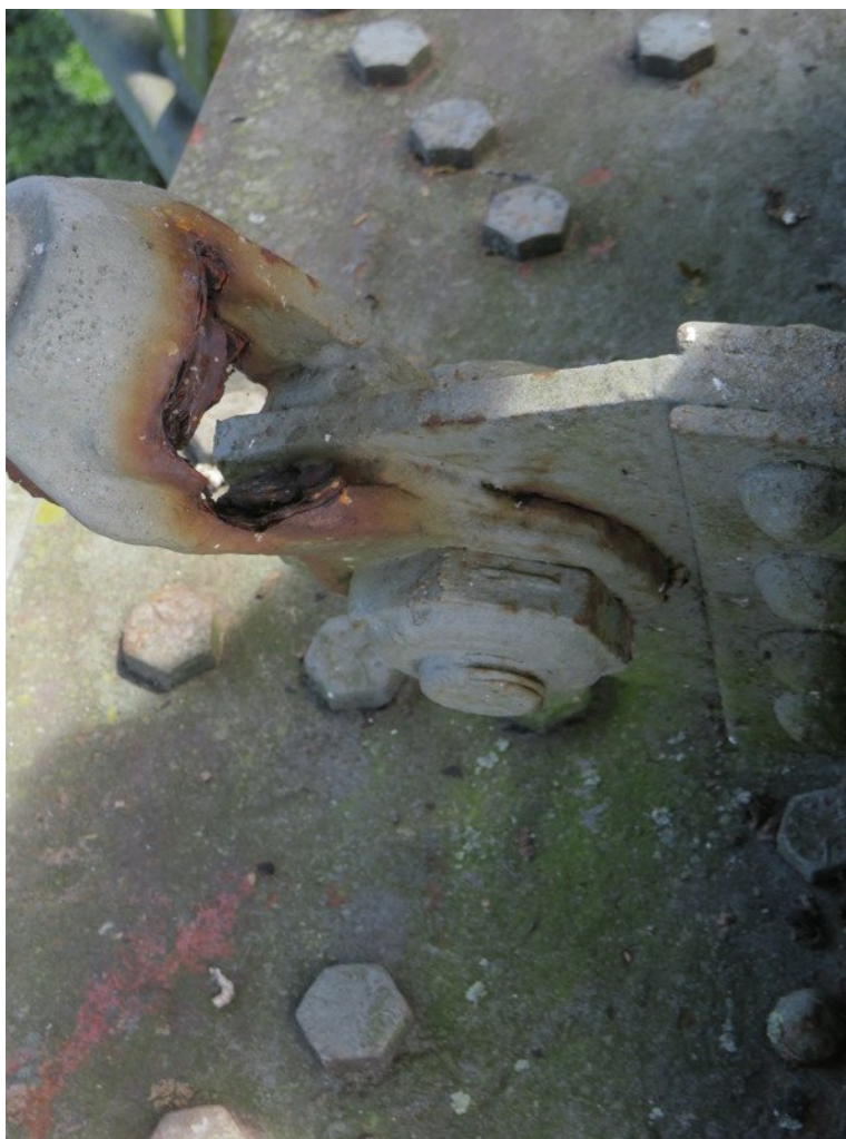
Cross bracing / diaphragms (Element 7): Corroded tie rod connection at UP T4.
