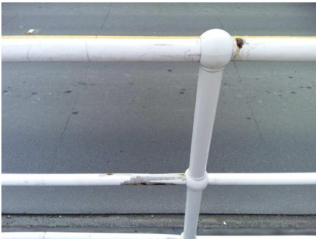
Painting: Barriers / Guardrails (Element 20): Loss of coating on traffic barrier. Upstream at L/4 from Cambridge end.
