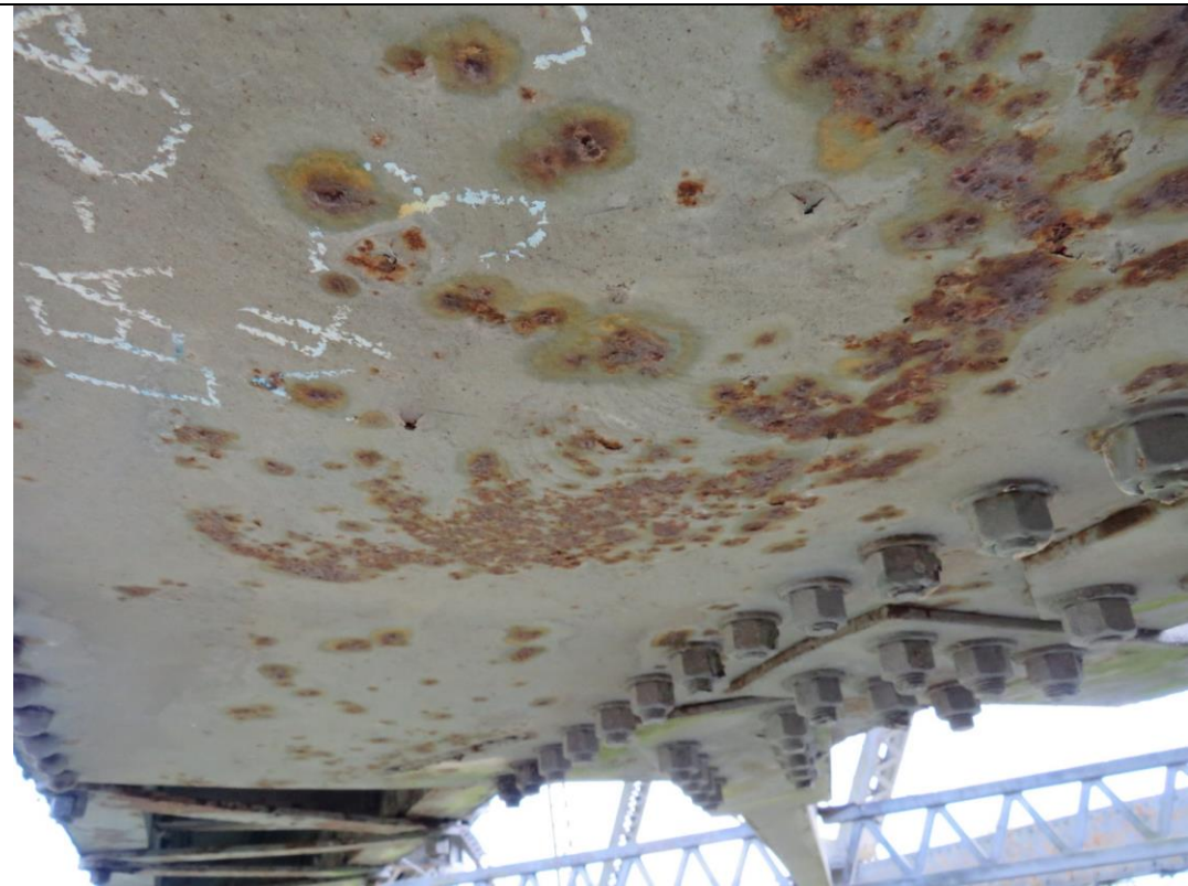
GENERAL CORROSION ON UDESIDE FACE OF BOTTOM ARCH
