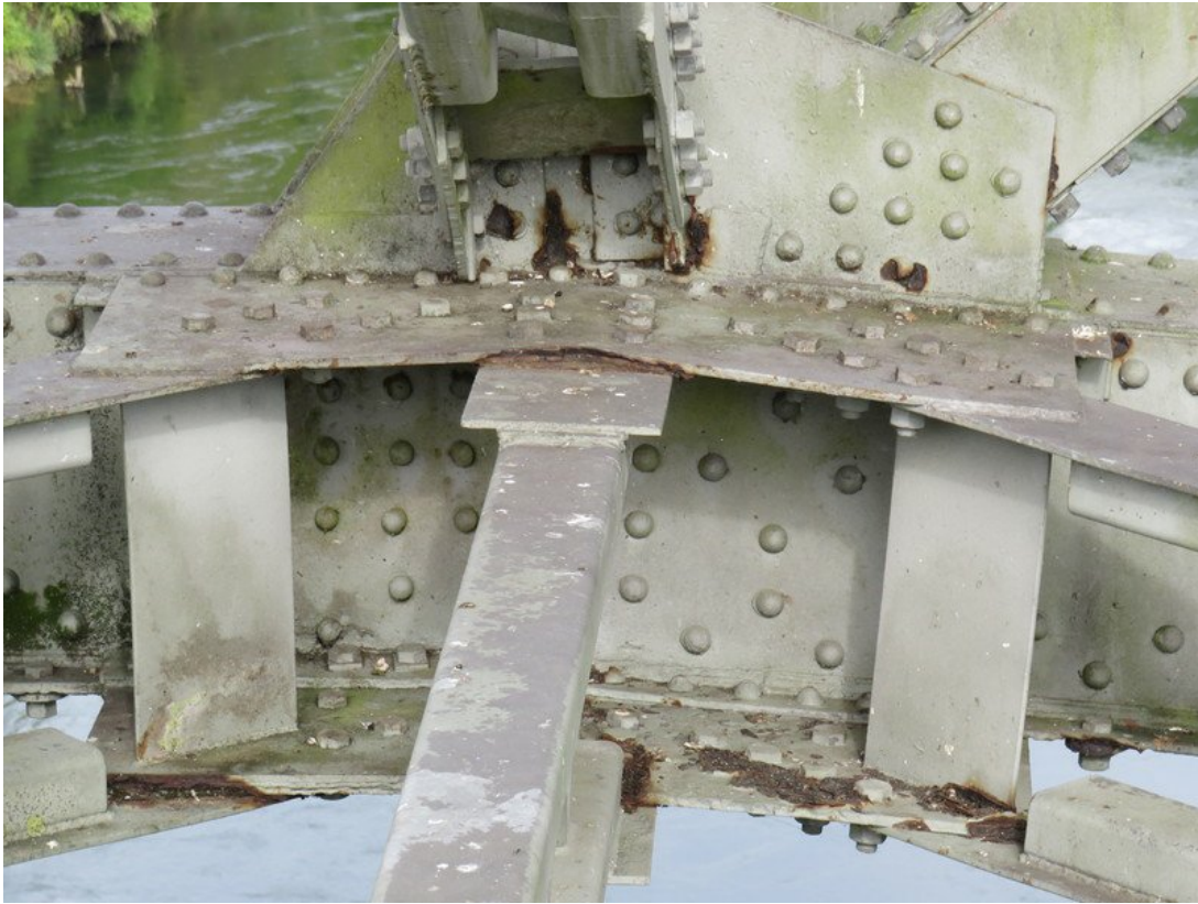
Primary Load Carrying Element (Element 1) : Element UB06-DN06 showing signs of delamination corrosion and loss of protective coating.
