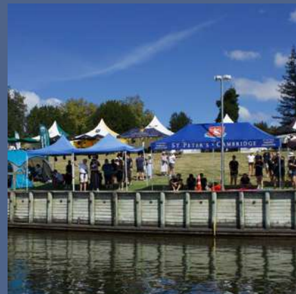
Grassed pedestrian access along the embankment with retaining wall that requires replacement
